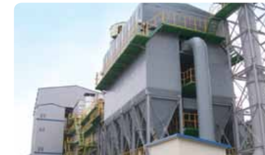
DCF Process applied to an Industrial Waste Incinerator in Mokpo
