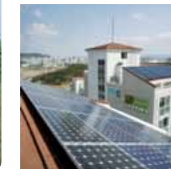
Installation in OKAM PRUGIO of Mokpo
